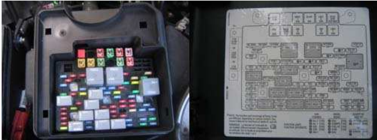
Pic 5 – Fuse Box with cover exposed
